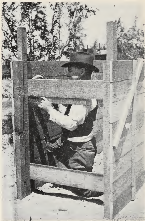
Fig. 9—Assembling side-wall forms and placing the 1×6-inch cross ties in the proper position.
